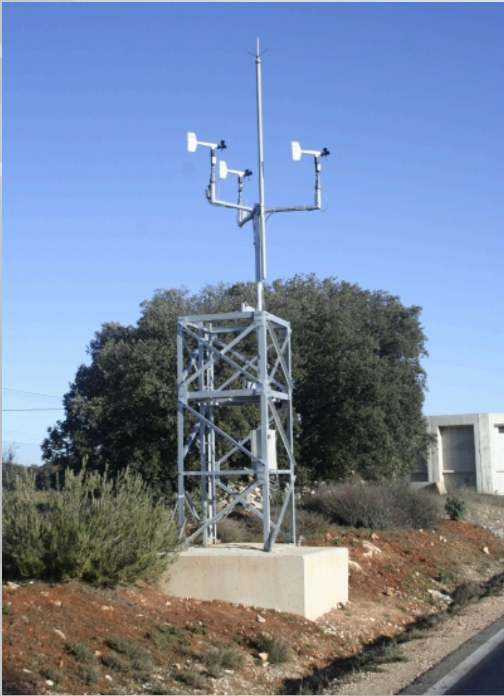
MONITORING FOR HIGH SPEED TRAIN-SPAIN
